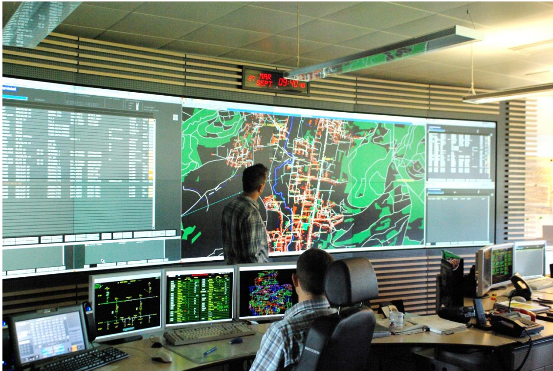
Photo 1: Dispatching centre Heisdorf (CREOS)
